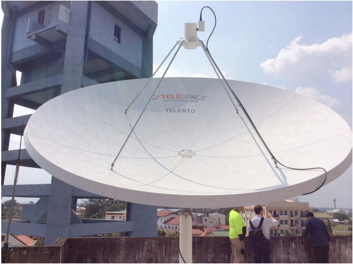
Installed and Operational Telesto System at the Laos DMH
